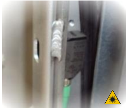
Closing obstacle detection cells located in the door risers. (about 6 cm above the threshold)
